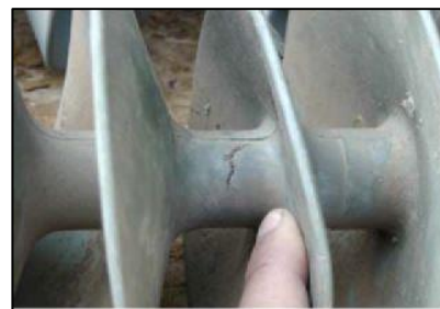
Fig. 10: Aged / Cracking Rubber
