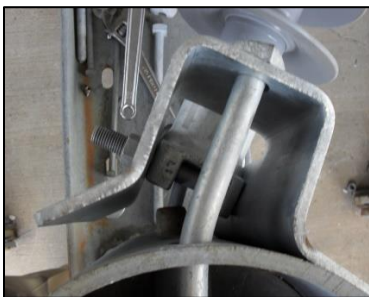
Fig. 7 – line post gain base, deformed due to longitudinal load
