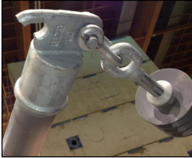
Fig. 8 – line post drop tongue fitting limiting this braced post assembly.
