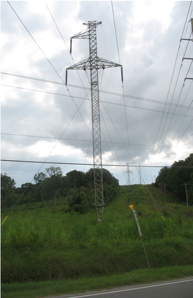
Tower Guy Application
